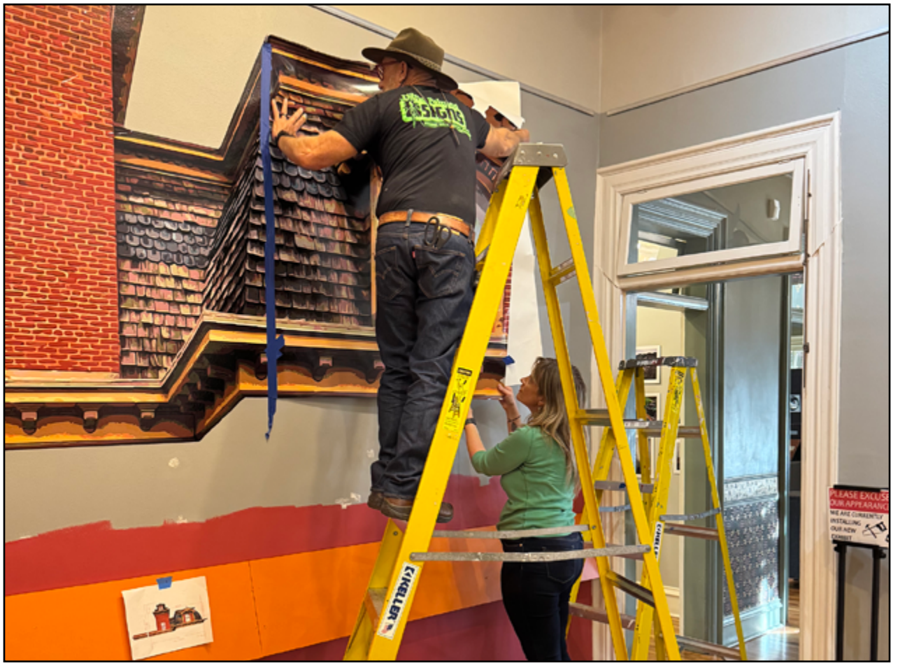
John and Jennifer Mahl of J&J Signs at work in December 2025, installing the large-format vinyl wall design for the museum’s latest long-term exhibit. The vinyl, typically used to wrap cars, offers both visual impact and lasting durability.
